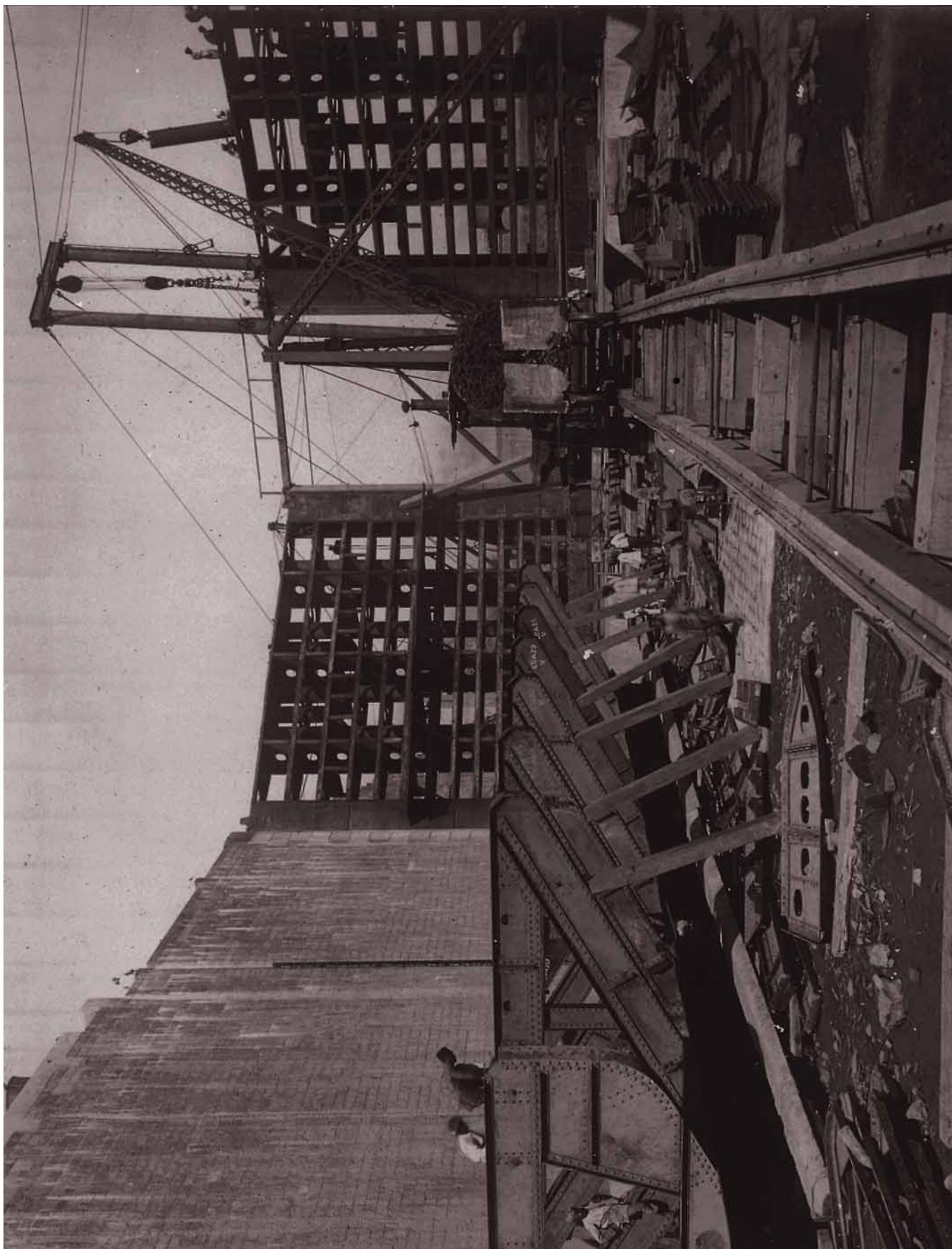
Inner gates of lock and dry dock caisson in course of erection. View looking towards north.
