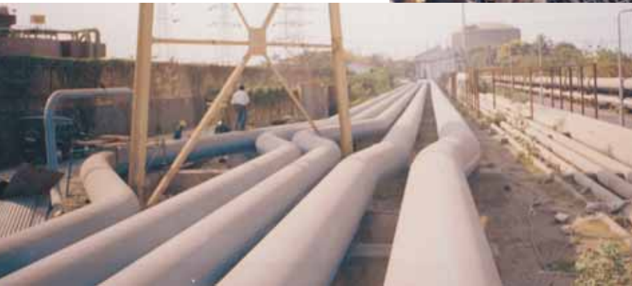
↑ View of pipelines between land fall point. & Pir Pau manifold
