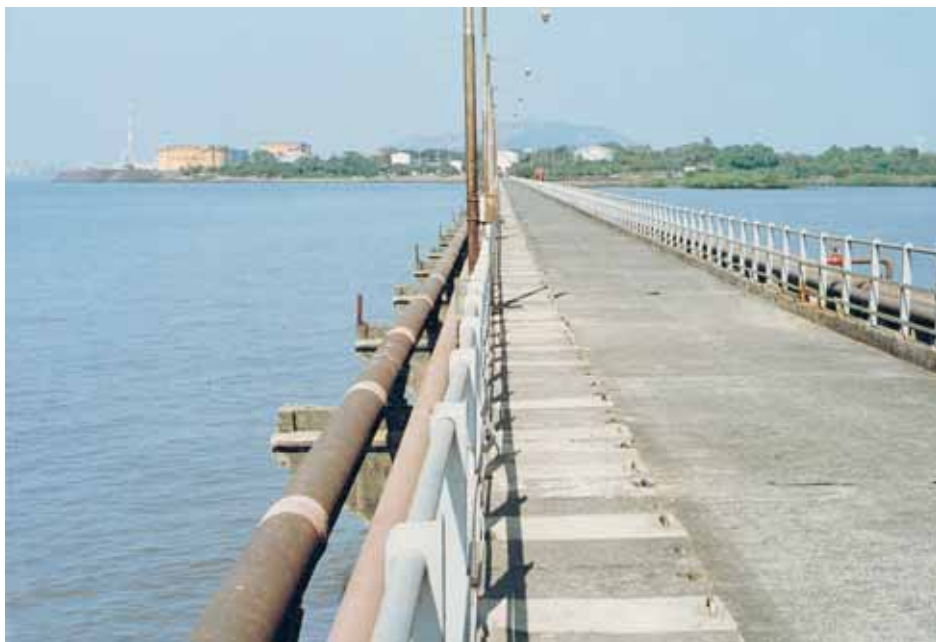
A view of approach trestle to Fourth Oil Berth at Jawahar Dweep with the island in the background.
