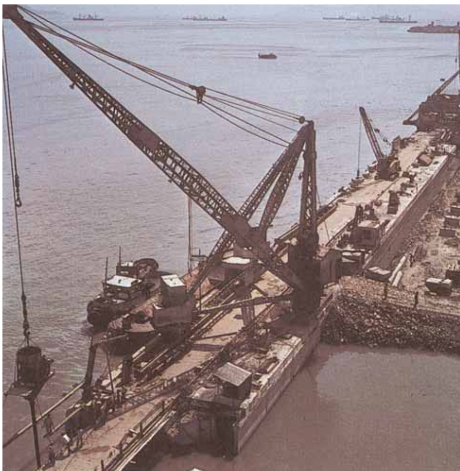
Work under way at Ballard Pier extension at Bombay Harbour involving precast buttresses bridged by 160T precast arch units.
