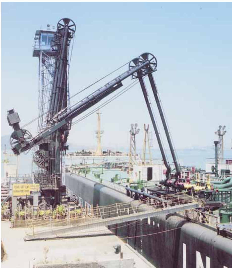
POL operations through loading arms (1997) at 4th oil berth Jawahar Dweep.
