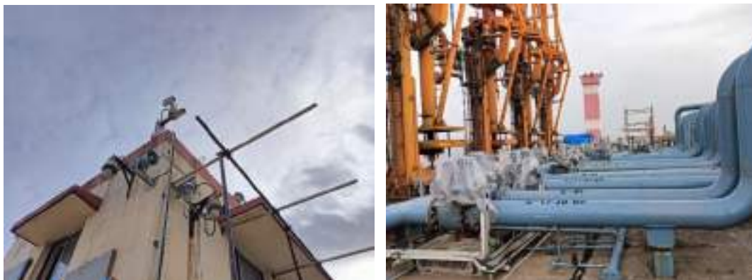
Figure 5.29 CCTV & Public Announcement System at Jetties (on the left), Jetty Manifold Pipelines, Valves and Marine Loading Arms (on the right)
