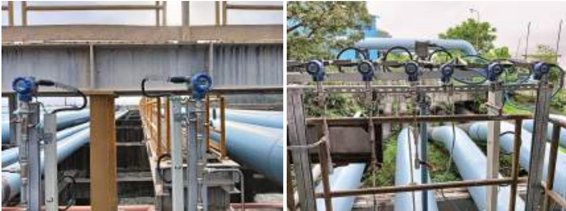
Figure 5.30 Pressure Transmitters / Temperature Transmitters on Oil Pipelines
