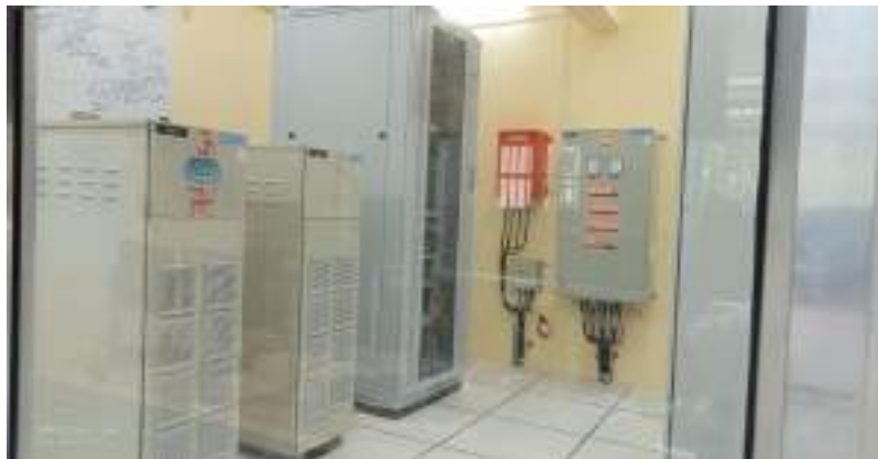
Figure 5.28 PLC System Panel at Marine Oil Terminal, Jawahar Dweep
