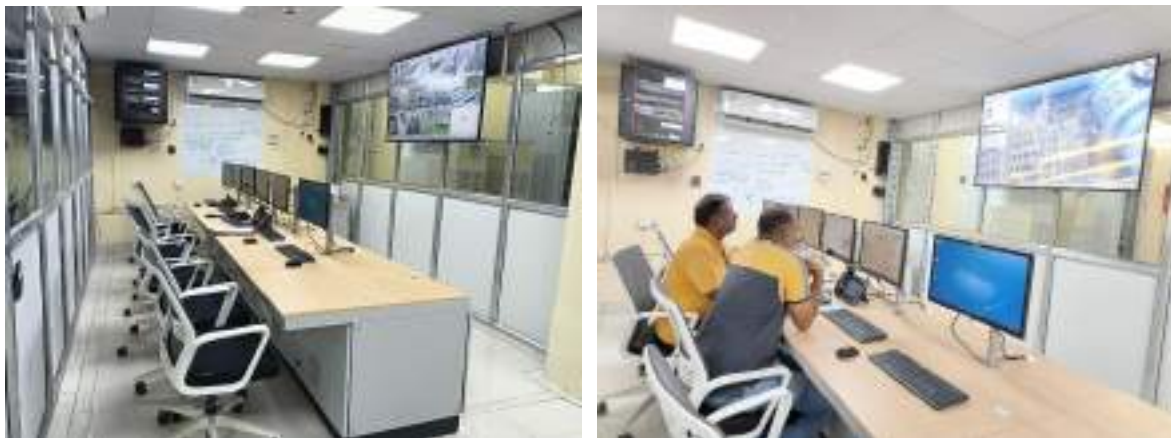
Figure 5.31 Master Control Room of SCADA at Marine Oil Terminal, Jawahar Dweep
